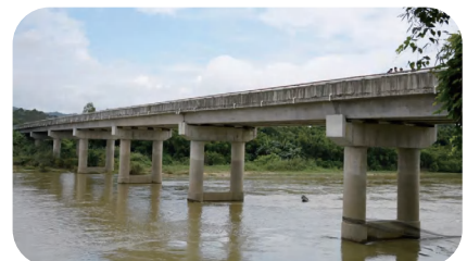
Bridge Pier Damage Detection
